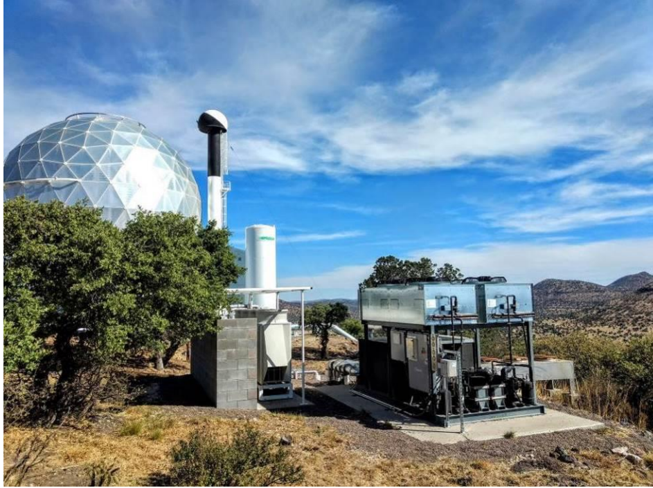
Figure 12. The 20 ton Advantage chiller supplies glycol to the Hobby Eberly Telescope from its location in the remote thermal site. (Photo taken by R. Spencer)
