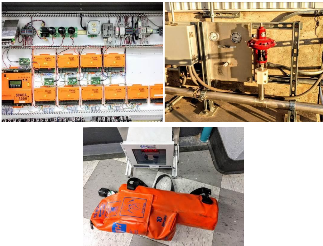
Figure 8. (Top Left) SCADA system, providing monitor and control functions of the VCSS. (Top Right) Nitrogen supply valve for the LNST. SCADA can send a command to shut down in emergency. (Bottom) Oxygen sensor will sound alarm if oxygen levels in location get to low. Some alarms will cause SCADA to send command to close main nitrogen supply valve. EEBA (Emergency Escape Breathing Apparatus) are located in numerous locations to allow personnel to escape if there is a nitrogen leak. (Photos taken by R. Spencer)
