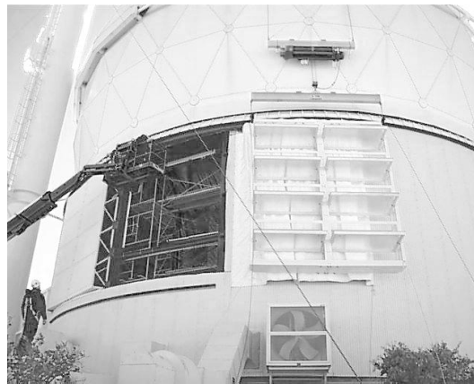
Figure 6: The custom hoist permitted accurate and safe positioning of the louvers for installation.
