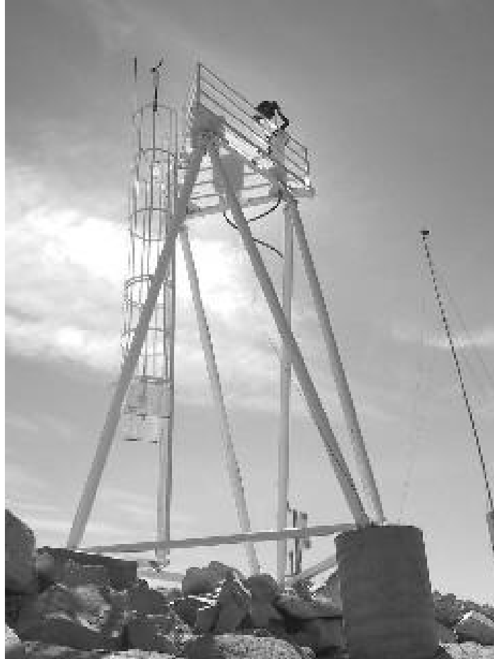
Figure 6: The DIMM platform at National Solar Observatory can experience a loss in stiffness at the top of the structure when a single pipe column is used for the telescope mount.
