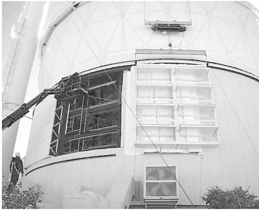
Figure 5: Louver crane in operation, preparing to install second louver module in the north side of the ring wall.
