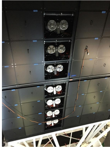
Figure 3. A full row of eight installed VIRUS units with the enclosure doors removed during installation. The VIRUS support structure (white weldment) is seen riding the air bearings at the bottom of the image. The black pipes seen above each unit remove heat from the controllers (seen between the cylinders of each unit.) (Image: T. Peterson)
